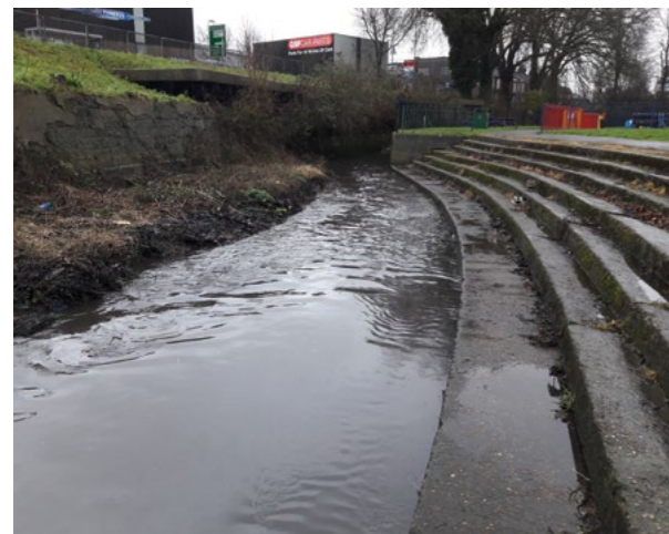
Manor Road Park, Luton prior to the river restoration works. The channel was constrained by concrete steps and a concrete riverbed [January 2018]
