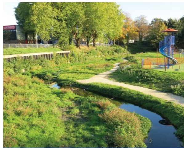
After river restoration work at Manor Road Park, Luton. The concrete steps have been removed and the channel has been naturalised and re-connected to the floodplain [September 2018]
